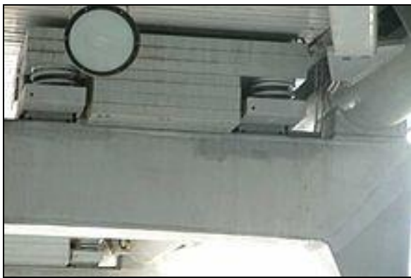
Fig 3: Dampers on the Bridge in London.
