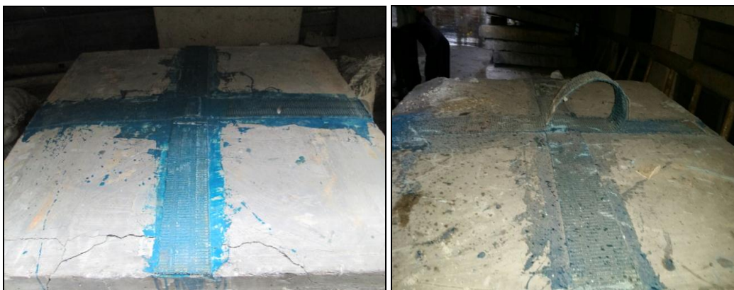
Fig 5: Crack pattern and debonding of the retrofitted slab.
